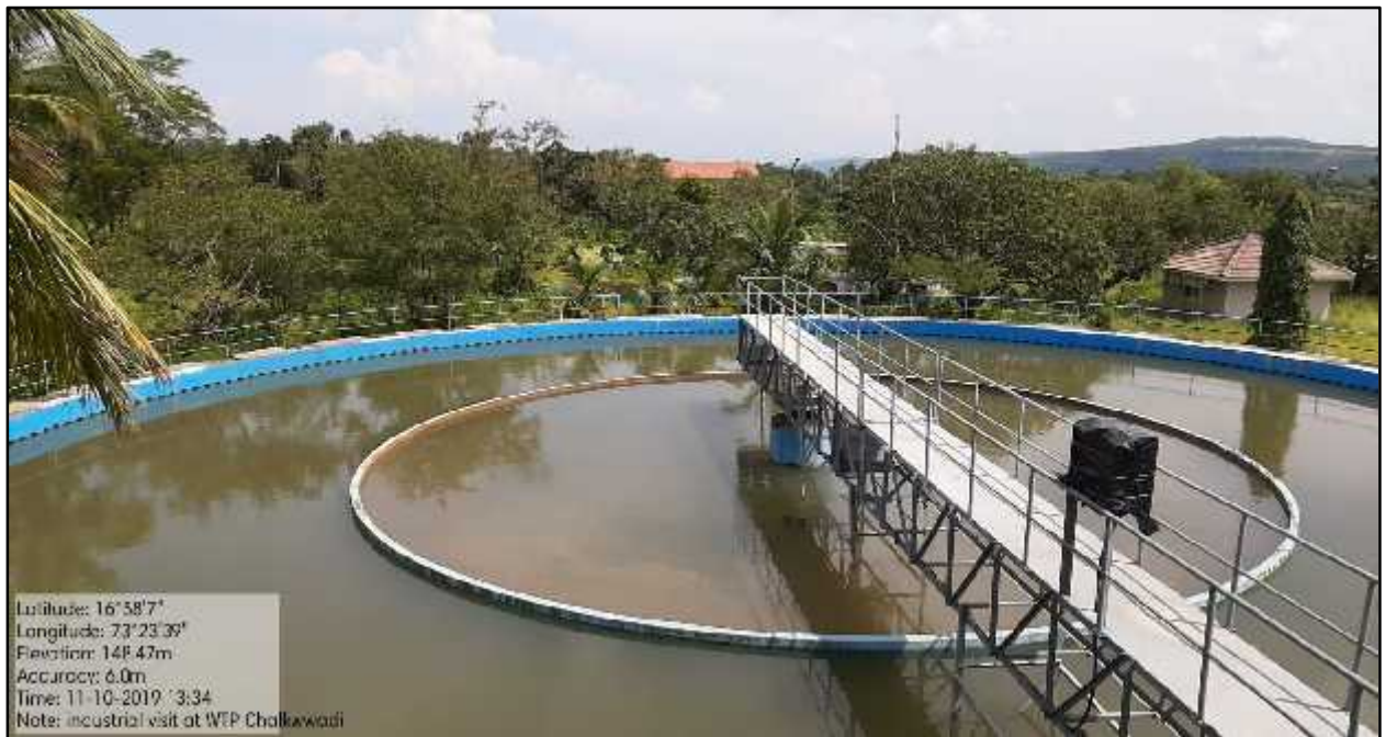
Sedimentation and Coagulation Tank
